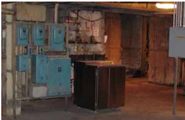
One of the hydrogen generators attached to the hydrogen manifold of one of the GE hydrogen-cooled generators at Mirant Mid-Atlantic's Dickerson, Md. power plant.
