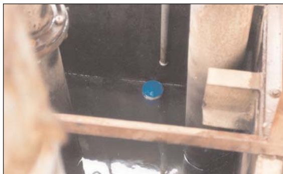
Figure 6. Storm water discharge interceptor
