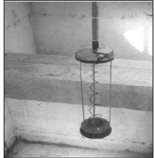
ID-223/500 installed in a flow stilling outlet tank, monitoring oil/water separator discharge.
