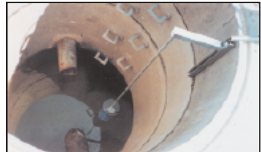
Leakwise ID-223 installed in a sump collecting water from a separator at a pipeline pumping station
